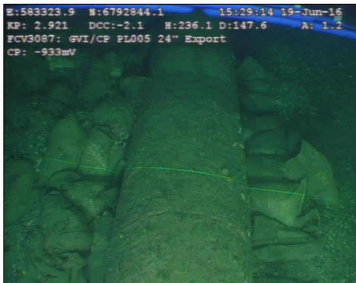
Figure 7-2 Typical Deposits (Pipeline Support) - 2016 Survey Footage
