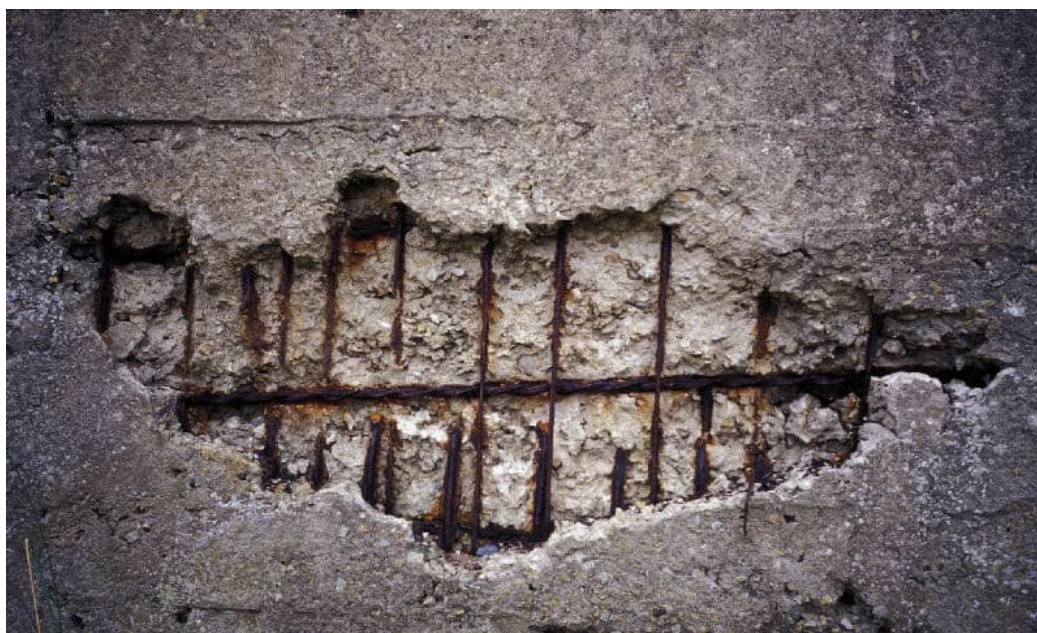
Figure 6-3: Example of Reinforced Concrete Spalling (not Dunlin Alpha)
