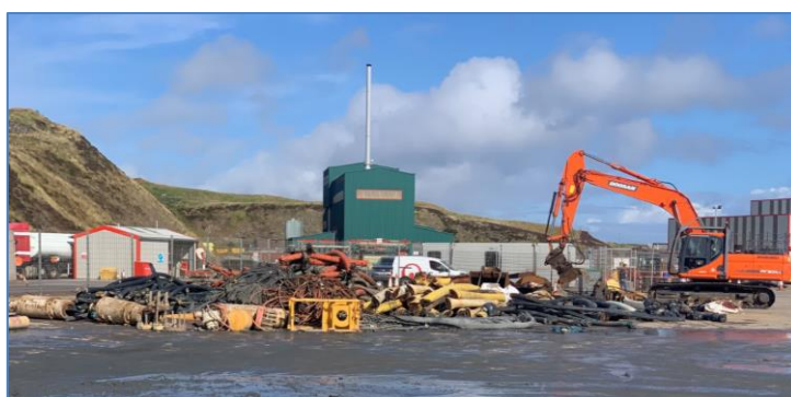
Waste Preparation & Separation
